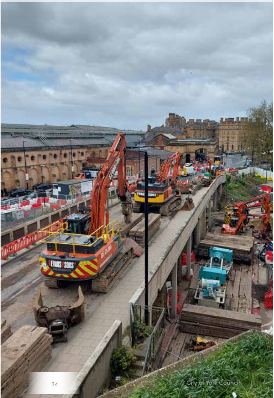
Figure 51 Delivering a major project at York Station Gateway: Preparatory work in advance of removing Queen Street bridge in spring 2024, to be replaced with a new station forecourt
